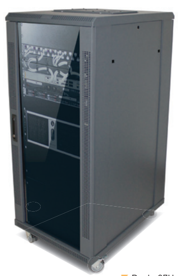
▲ Rack 27U (Mounted and adjusted)
